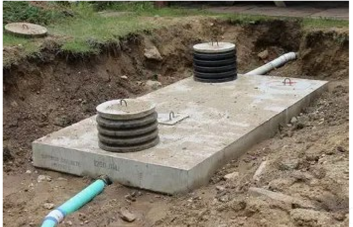
Septic Tank | greenhavenrealty.com
