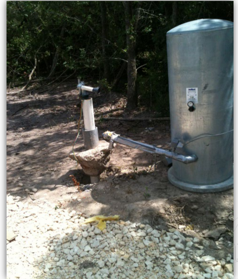
Damaged Private Well
